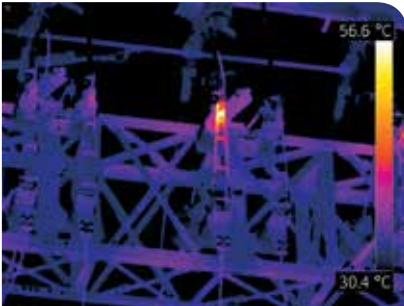
Overheating substation circuit breaker
